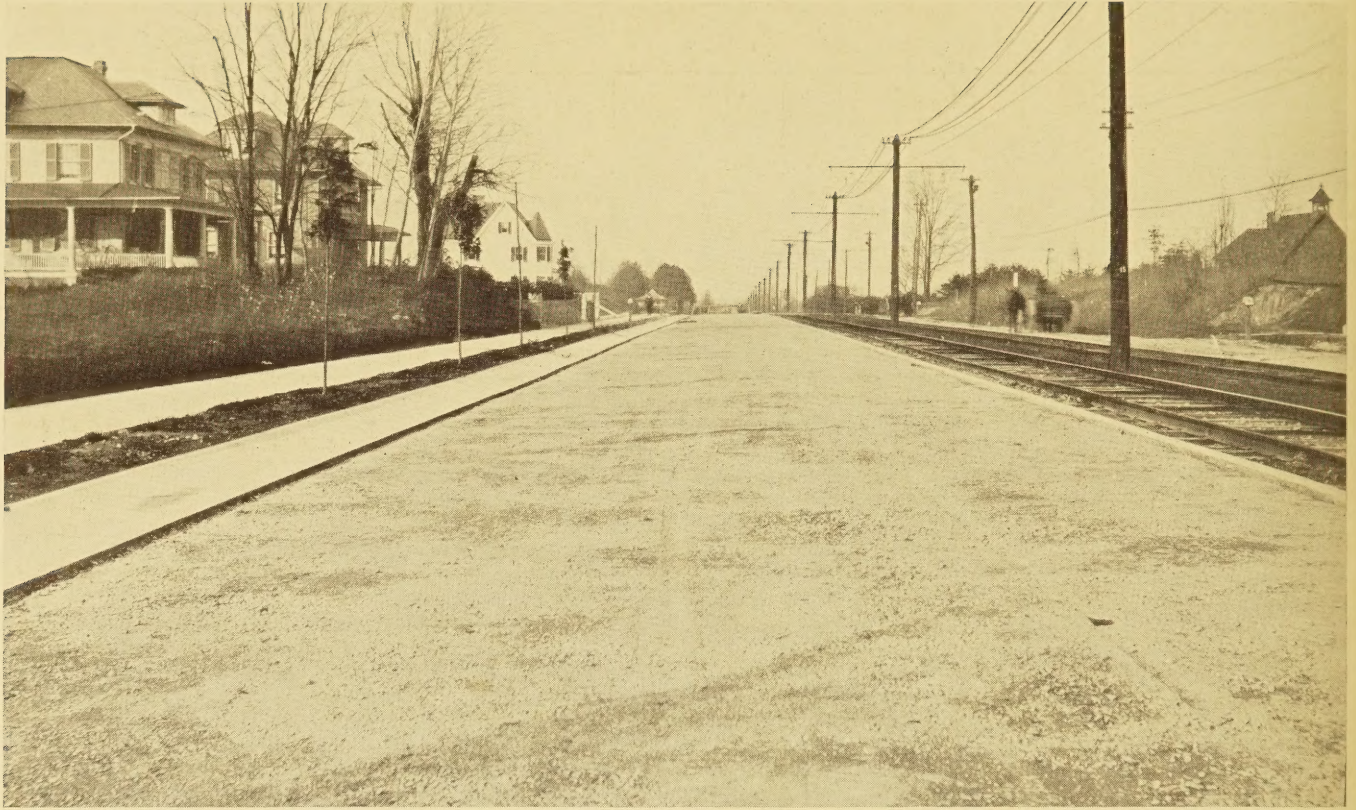
CONNECTICUT AVENUE EXPERIMENTAL ROAD, CHEVY CHASE, MD., NOVEMBER 11, 1912 PORTLAND CEMENT CONCRETE BASE READY FOR CONSTRUCTION OF BITUMINOUS CONCRETE SURFACE
